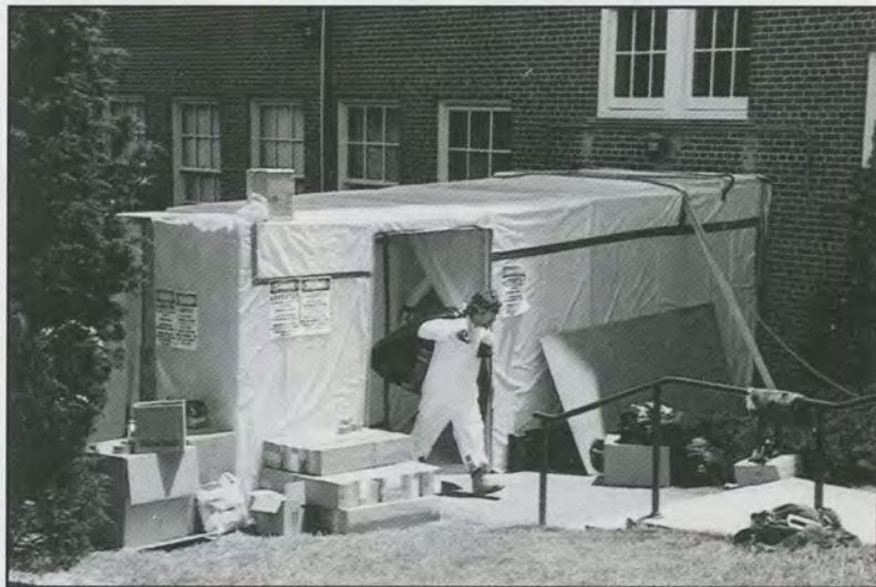
The asbestos containment tent attached to Kellenberg during the asbestos clean-up and removal process.
